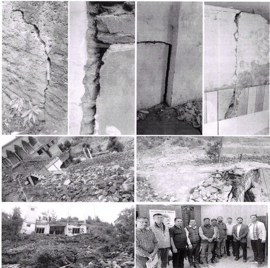
Figure 3: Cracks observed in the various structures of the affected areas. The lower right panel shows the committee members with the Conservator of Forests, Chenab Circle, Jammu and Kashmir.
